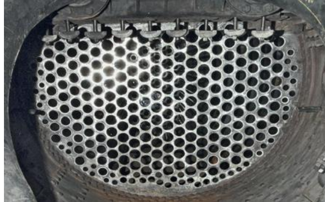
Boiler tube sheet
