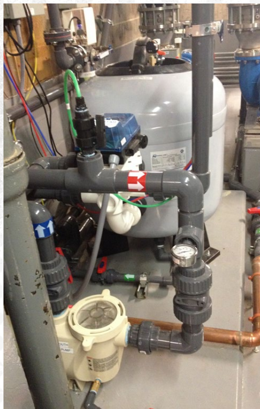
Water Feature Pumps & Pump Stations.
