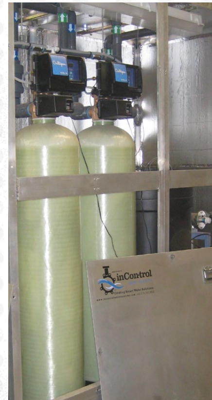
Water Quality Components capturing debris, sediment, and treating mineral contents.
