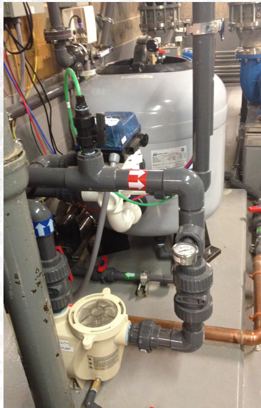
Water Feature Pumps & Pump Stations.
