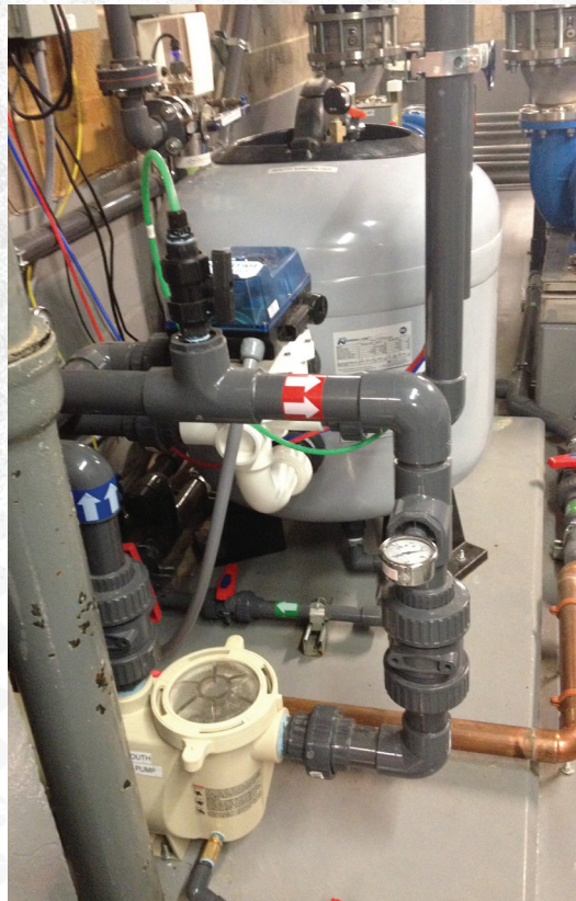
Water Feature Pumps & Pump Stations.
